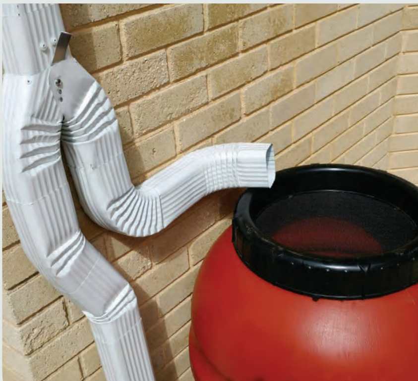
This diverter has a flap at the top, which can be switched to allow flow to go into the rain barrel (right downspout) or flow through the downspout onto the ground (left downspout).
