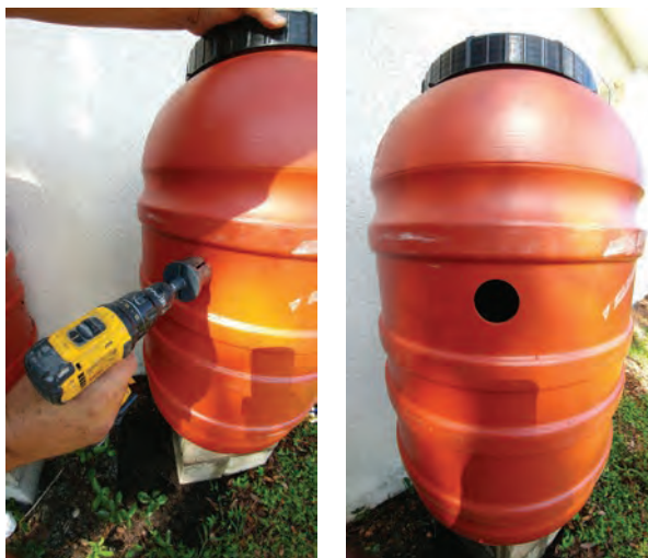
Drill a hole in each barrel for a connector. For a two-inch PVC male adapter, a 2-3/16-inch hole saw was used. Pick a flat spot on each barrel so connection is level.
