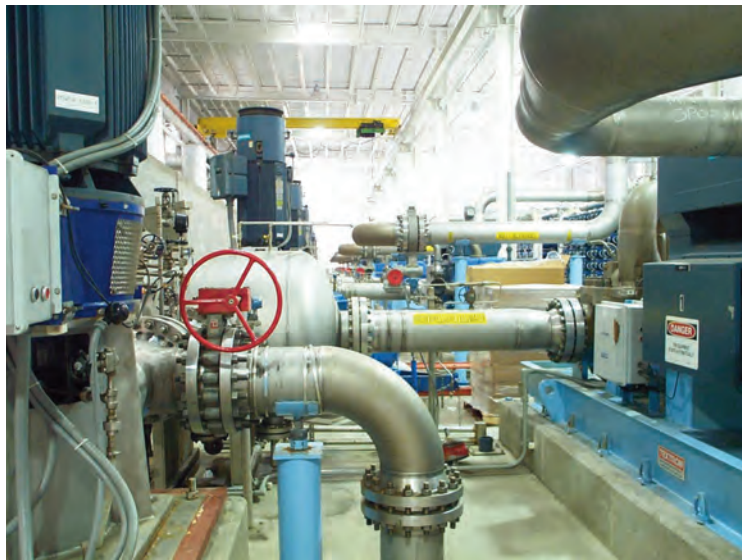
An interior view of the Tampa Bay Seawater Desalination facility.
