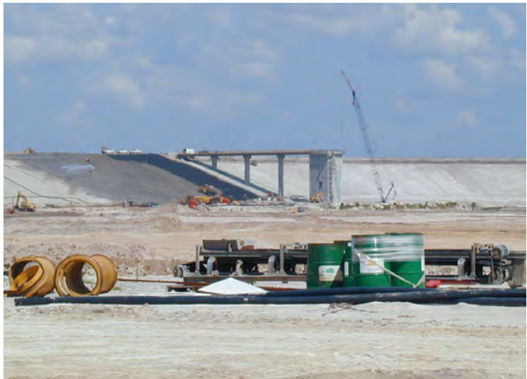
Tampa Bay Water’s C. W. Bill Young Regional Reservoir during the construction phase.
