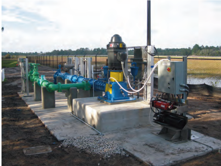
A typical aquifer storage and recovery well.
