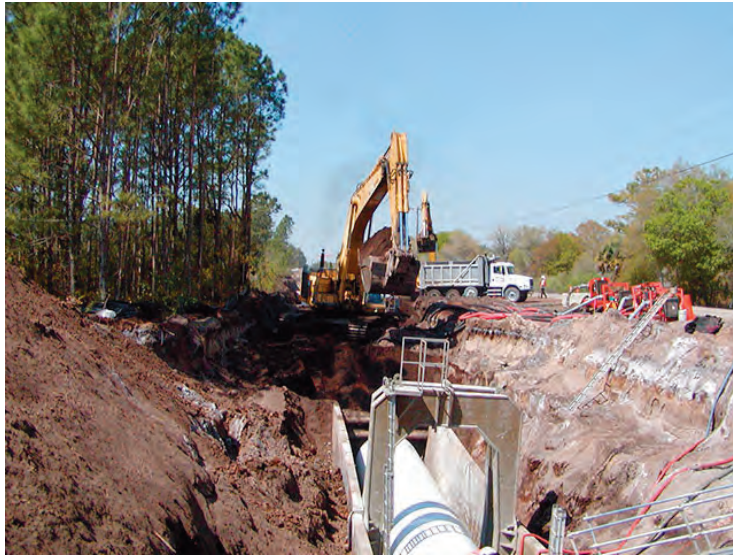
Construction of a major potable water transmission pipeline for Tampa Bay Water.
