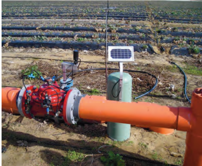
Solar-powered, remotely operated valves on an irrigation system enhance the efficiency of irrigation events, which reduces water use.
