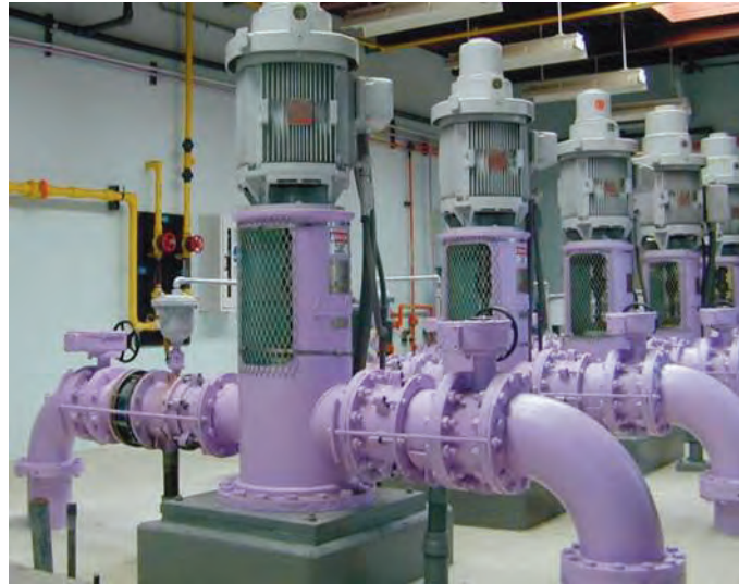
The District has provided hundreds of millions of dollars in matching funds to local governments to develop water supply infrastructure such as this reclaimed water pump station.
