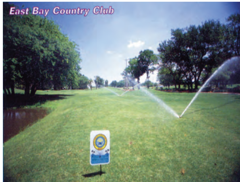
The District has partnered with many utilities in Pinellas County to develop projects to irrigate golf courses with reclaimed water.
