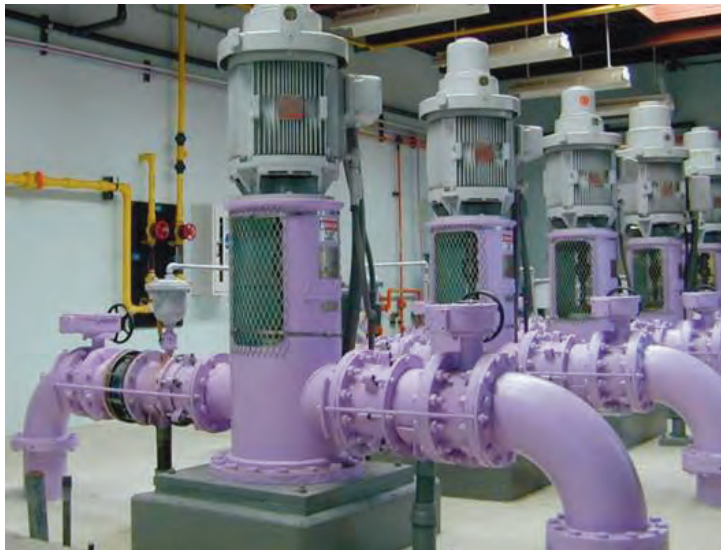
A reclaimed water pump station.
