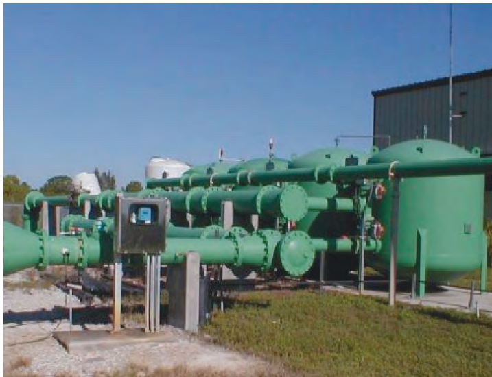
The pre-filtration system of a brackish groundwater desalination facility.
