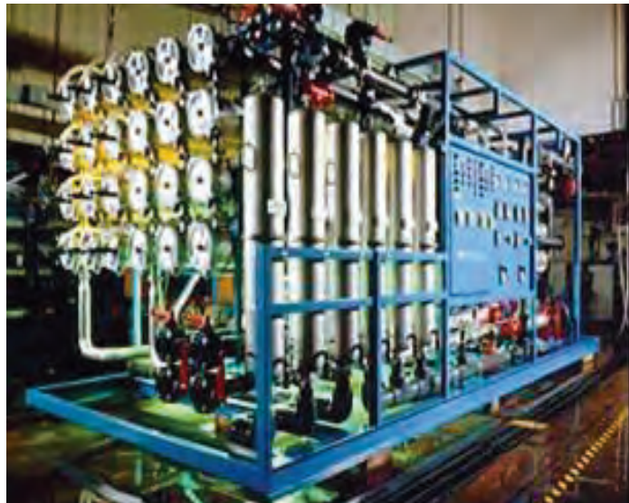
Reverse osmosis membranes in a brackish groundwater treatment facility.
