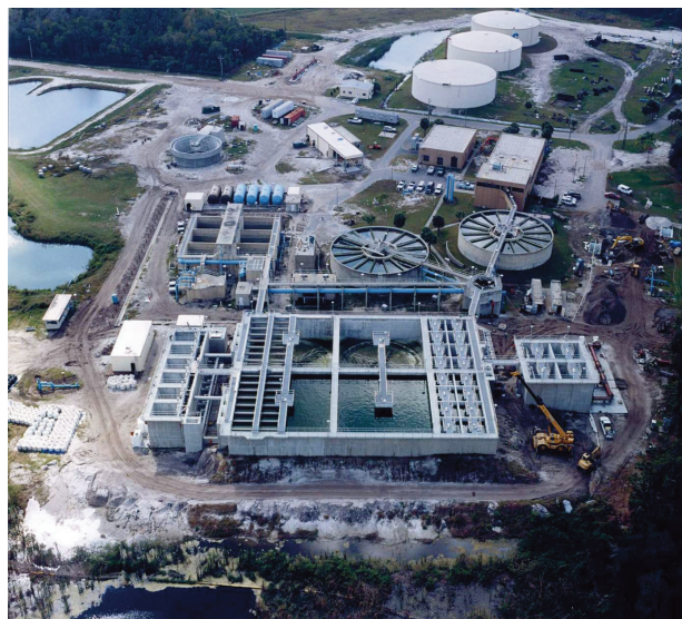
Construction of an early phase of the Peace River Manasota Regional Water Supply Authority's water treatment plant.
